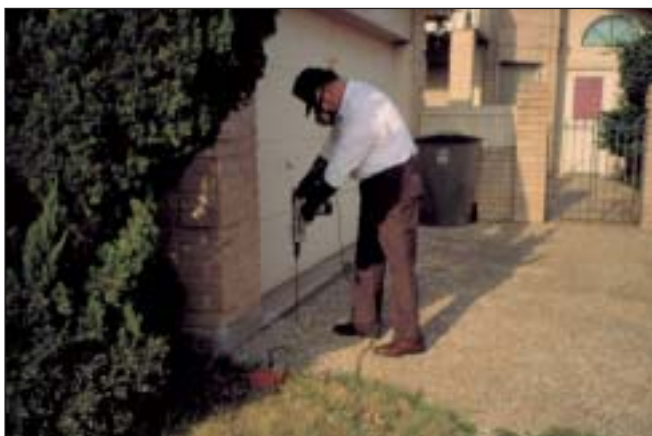
A rotary hammer drill is used to drill holes for the sub-slab method of termite treatment.
